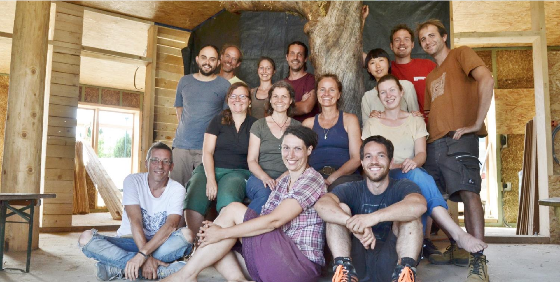
Building Site Workshop St. Georgen in Lavanttal 2019 / Carinthia/Austria Straw Bale Infill, Clay Plaster, Reciprocal Roof (with Okambuva)
