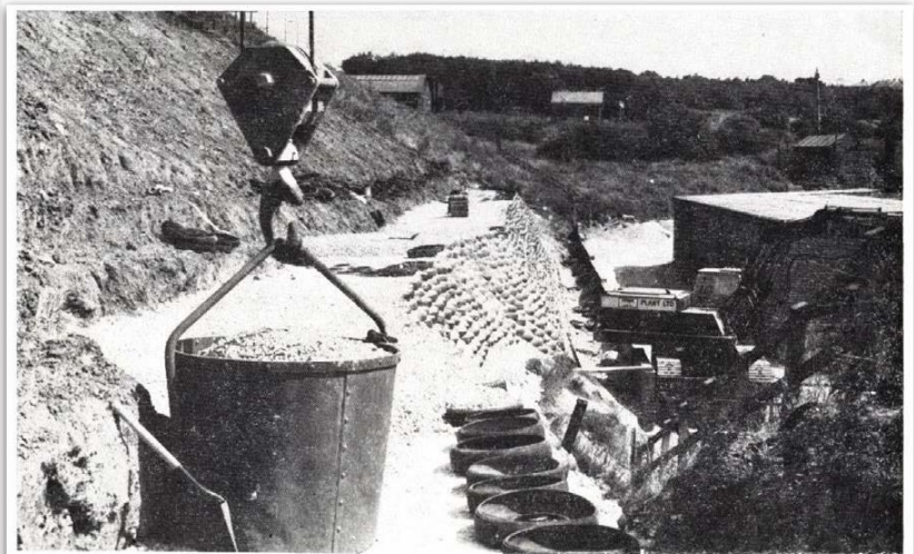
Fig. 4. During construction, Crusher run had to be treble handled using the Poclair for the lower section and the skip for the upper section. Final placing was by hand shovel
